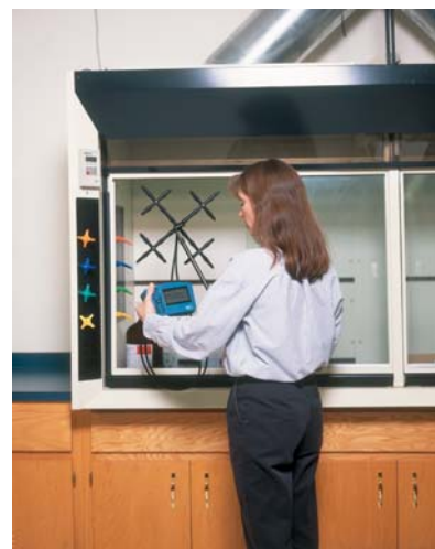
Figure 15. Face velocity is the primary method of evaluating fume hood performance after initial set-up.
